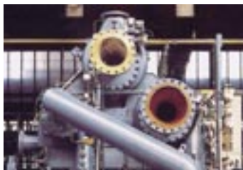
Picture 13.1: Intake control device
